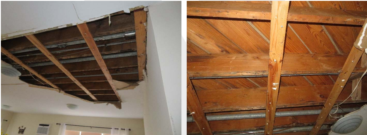
Figure 5. Summary of observations made in Unit 209: Exposed ceiling framing below recent water leak from roof drain (left); closeup indicating termite damage to floor joists (right).
