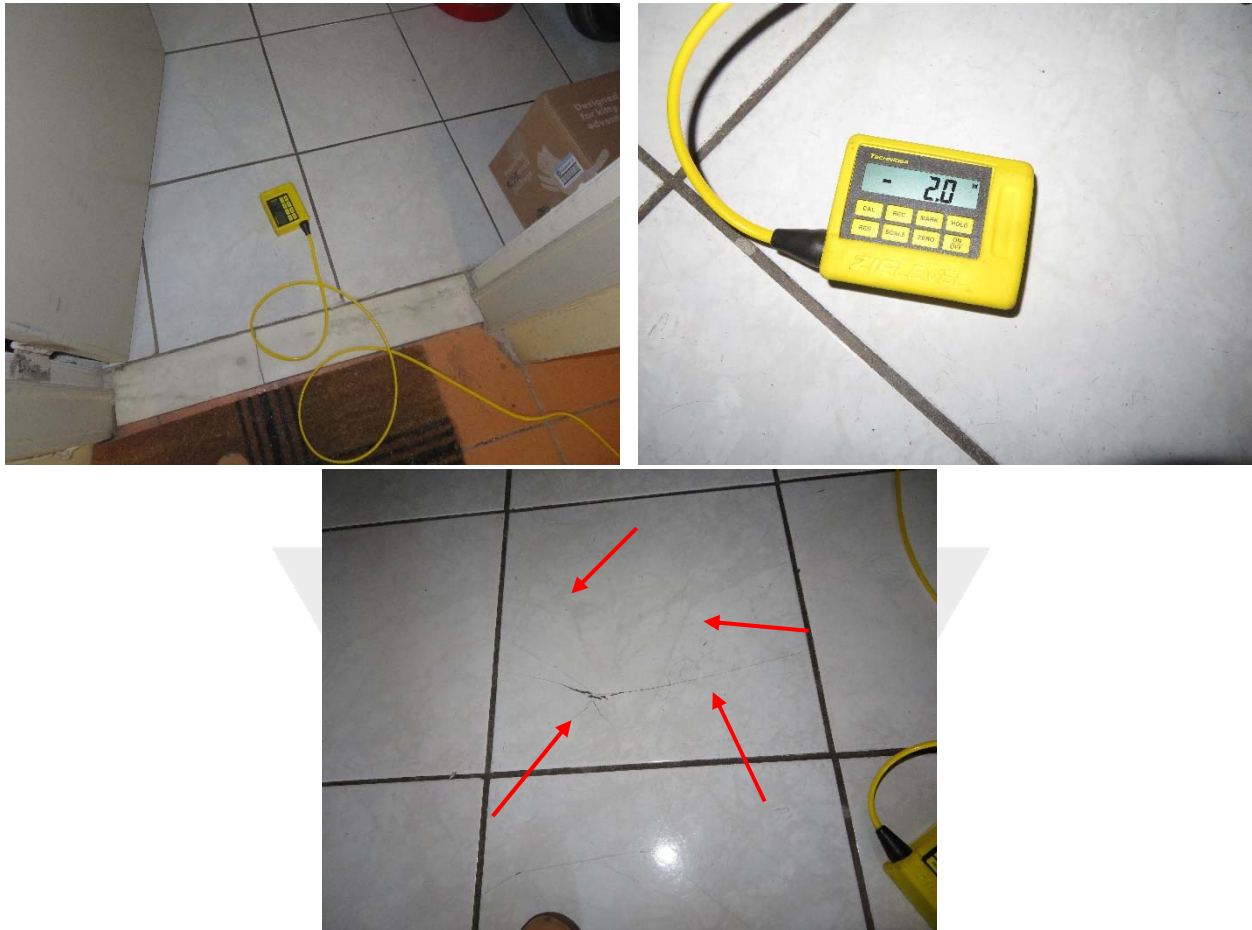
Figure 2. Summary of observations made in Unit 310: Relative elevation measurements taken with ZipLevel ( top row ); cracks in ceramic tile flooring installation in middle of living room ( bottom row ).
