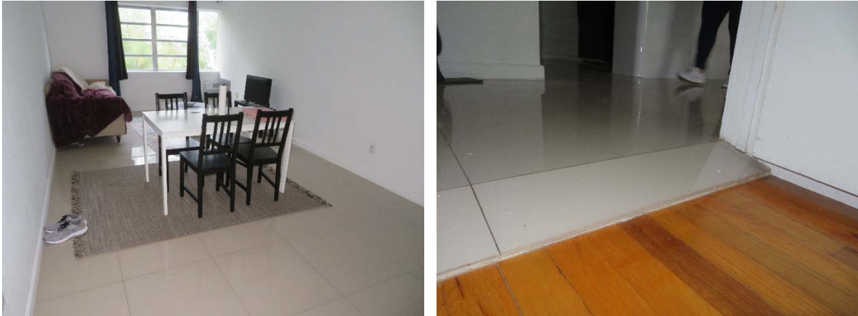
Figure 4. Summary of observations made in Unit 307: Installation of ceramic tile flooring within living room (left); termination of ceramic tiles at bedroom entrance, noted by ramp constructed (right).
