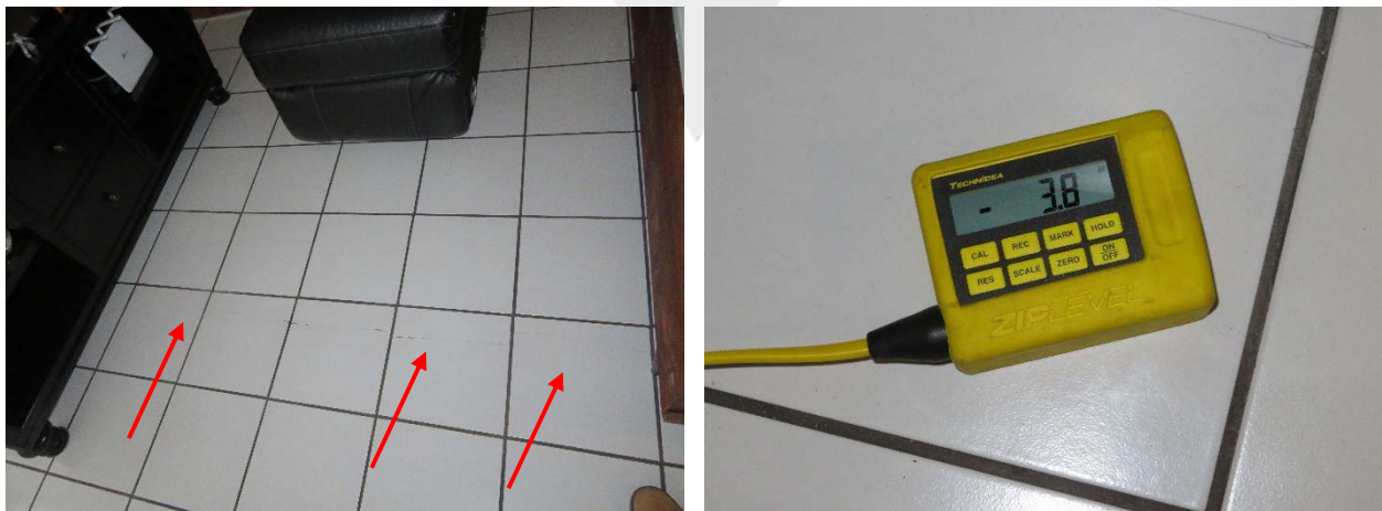
Figure 3. Summary of observations made in Unit 308: Linear crack in ceramic tile flooring installation extending across living room ( left ); relative elevation measurement taken with ZipLevel ( right );.
