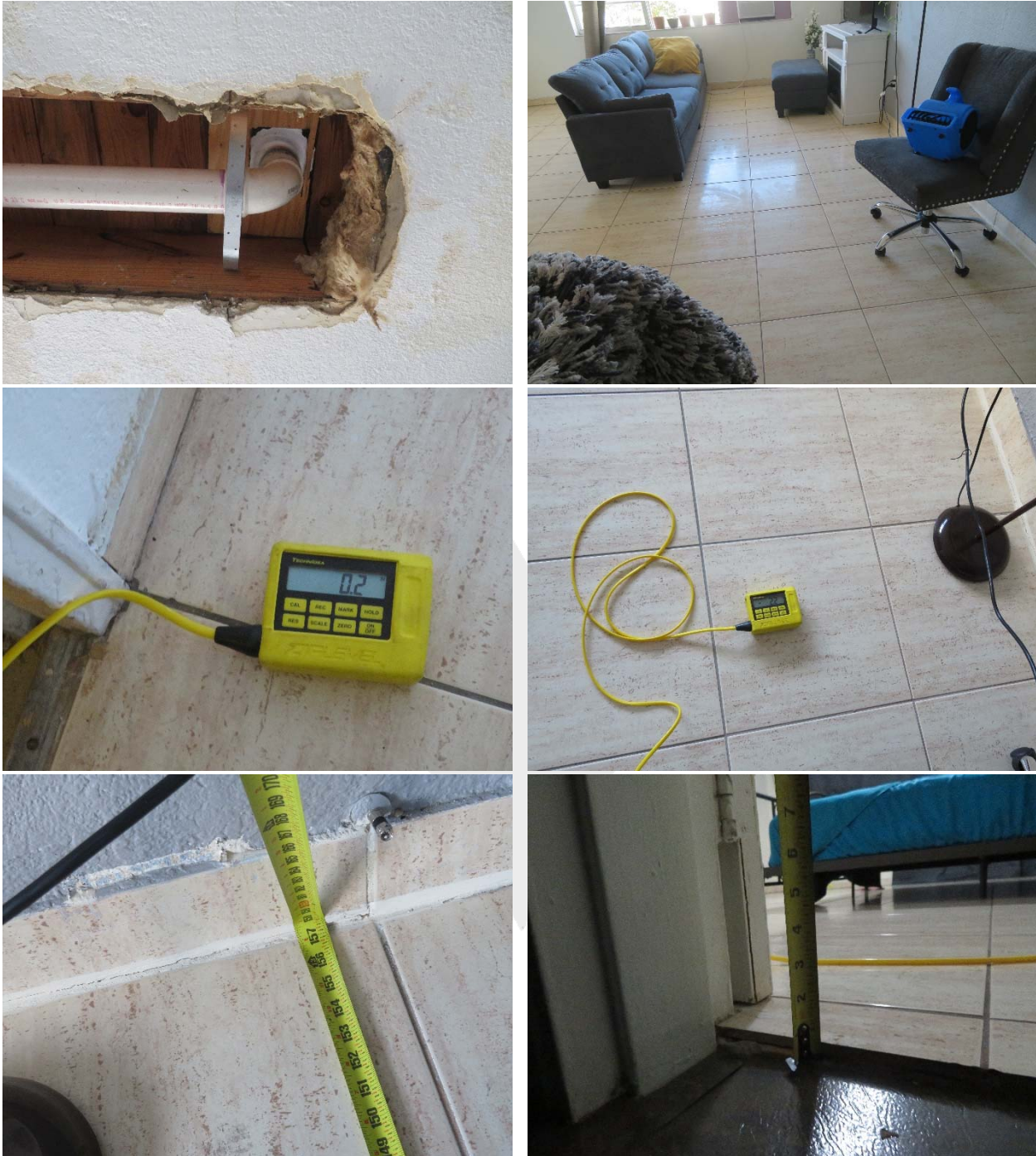
Figure 1. Summary of observations made in Unit 309: Collapsed section of ceiling drywall under roof drain ( top-left ); Overview of sagging floor in living room ( top-right ); relative elevation measurements taken with ZipLevel ( middle row ); measurement of presumed joist span of 13 feet ( bottom-left ); ceramic tile flooring installation over wood decking ( bottom-right ).
