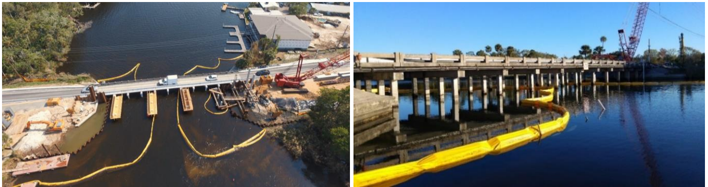
Figure 1. Halls River Bridge under construction (a) and existing bridge before demolition (b). [Courtesy of Astaldi Construction Corporation]
