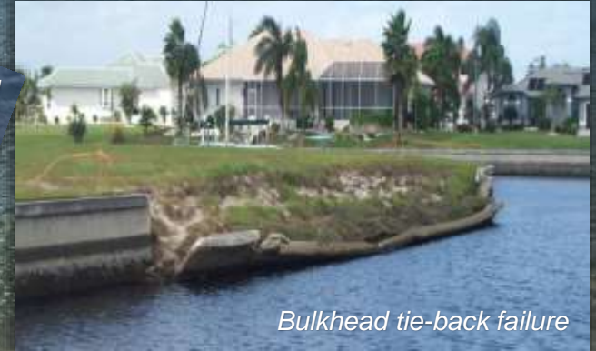
Bulkhead wall panel failure
