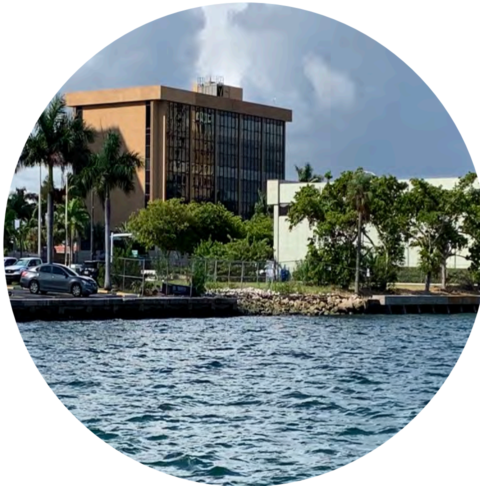
Seawalls at different states of repair
