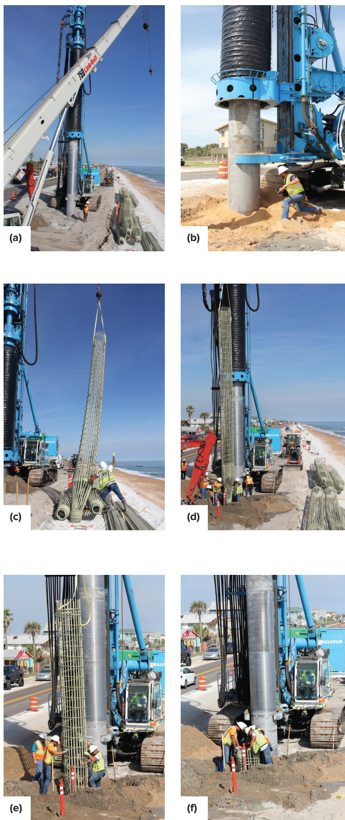
Fig. 6: A specialized drill rig was used to install the secant piles using the cased auger-cast method. The installation sequence comprised: (a) drilling; (b) soil removal and grouting; (c) GFRP cage lifting; (d) cage alignment; (e) cage insertion into the grout; and (f) final cage positioning
