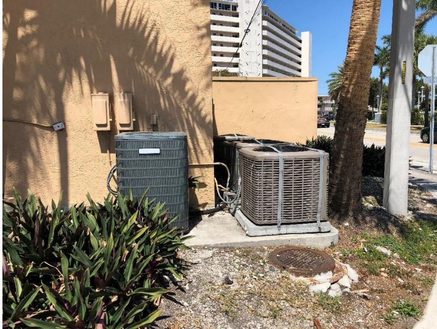
HVAC units in the eastern portion of the subject Site.
