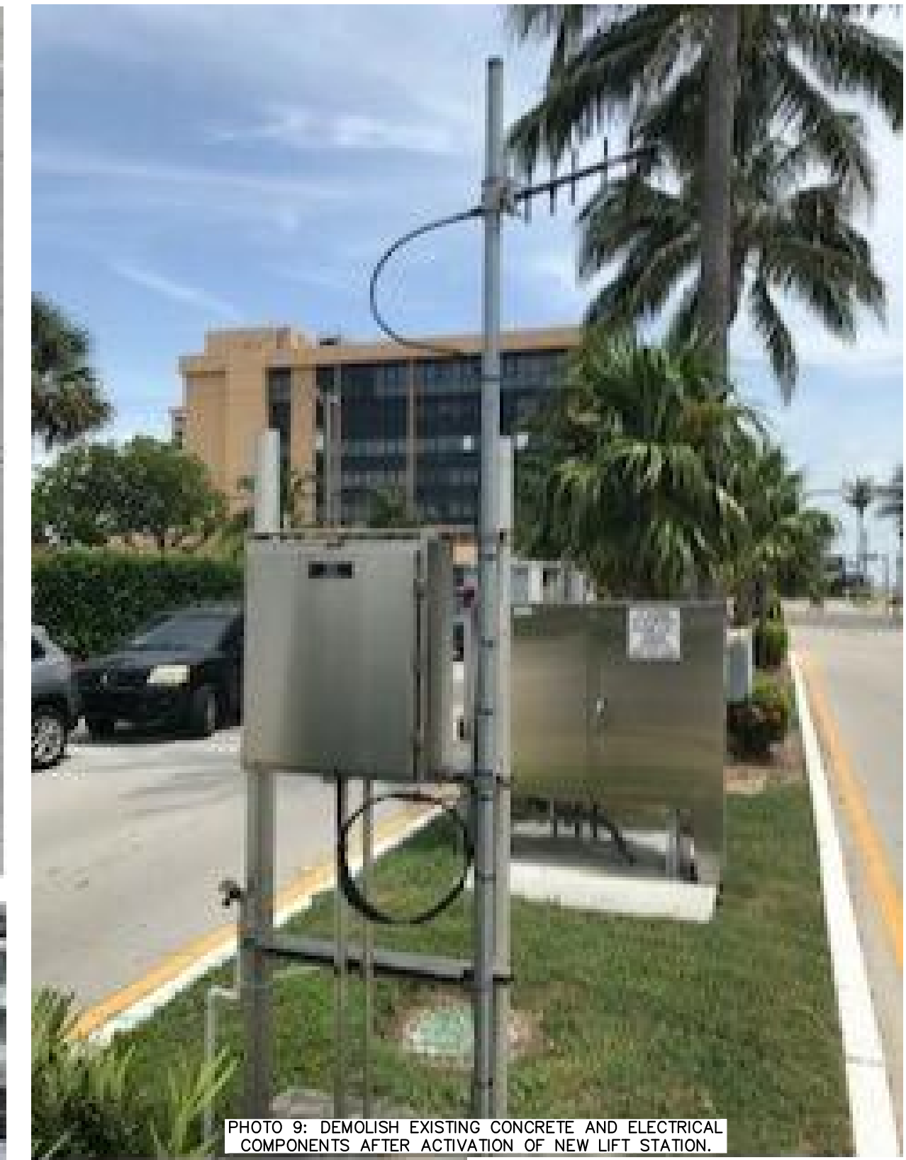
PHOTO 9: DEMOLISH EXISTING CONCRETE AND ELECTRICAL COMPONENTS AFTER ACTIVATION OF NEW LIFT STATION.
