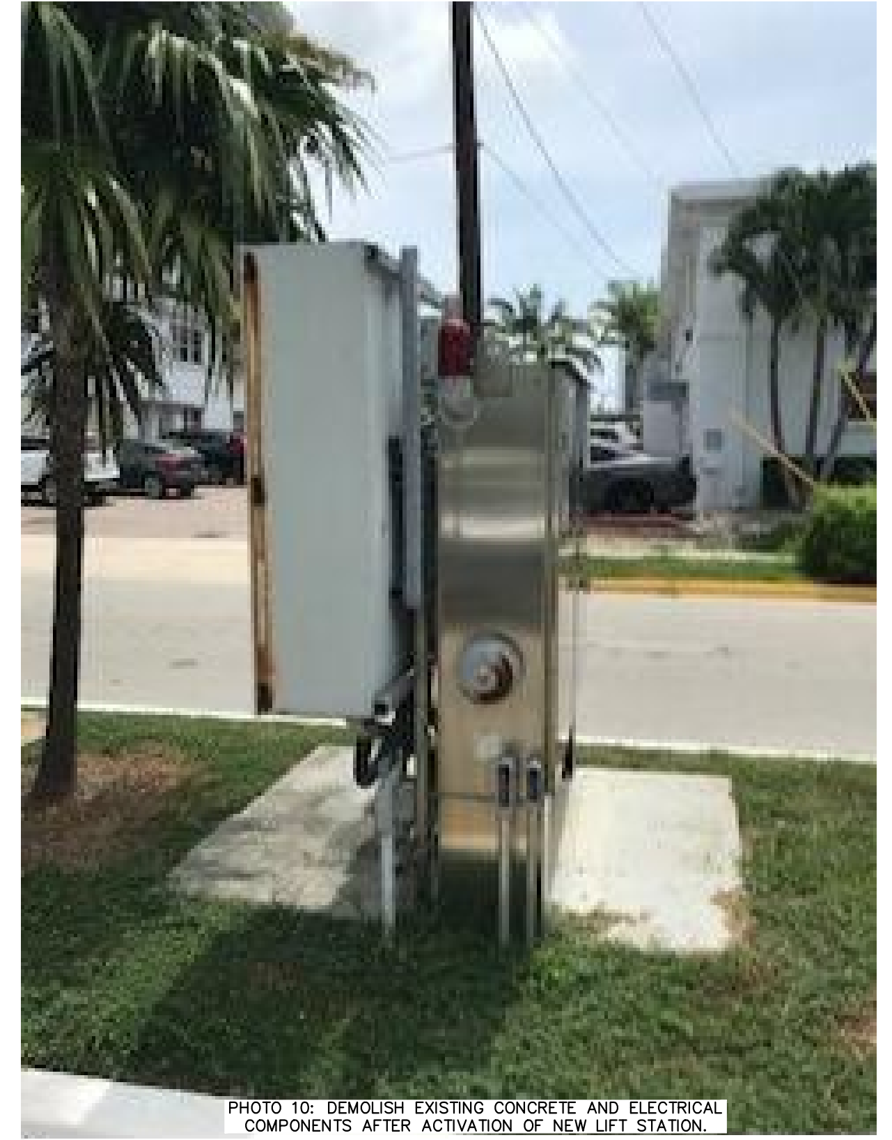
PHOTO 10: DEMOLISH EXISTING CONCRETE AND ELECTRICAL COMPONENTS AFTER ACTIVATION OF NEW LIFT STATION.
