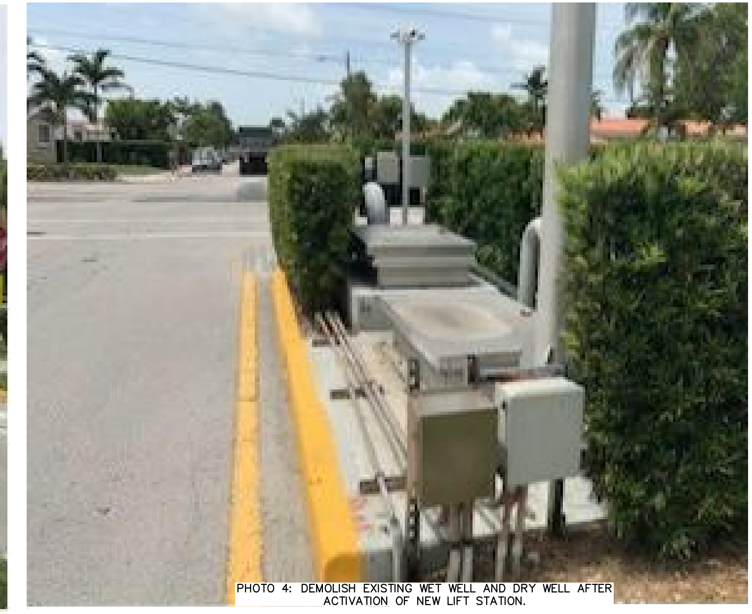
PHOTO 4: DEMOLISH EXISTING WET WELL AND DRY WELL AFTER ACTIVATION OF NEW LIFT STATION.
